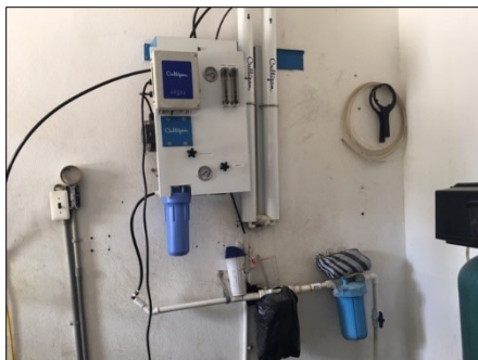
Water Purification System
